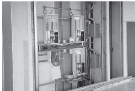
Figure 12.18 Electrical riser on office floor level
