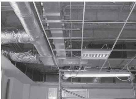
Figure 12.22 Services in ceiling void
