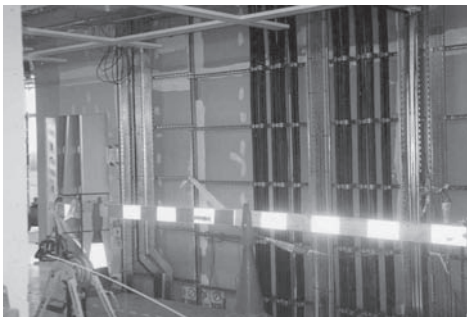
Figure 12.17 Incoming electrical riser
