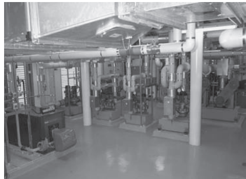
Figure 12.12 Typical heating plant room
